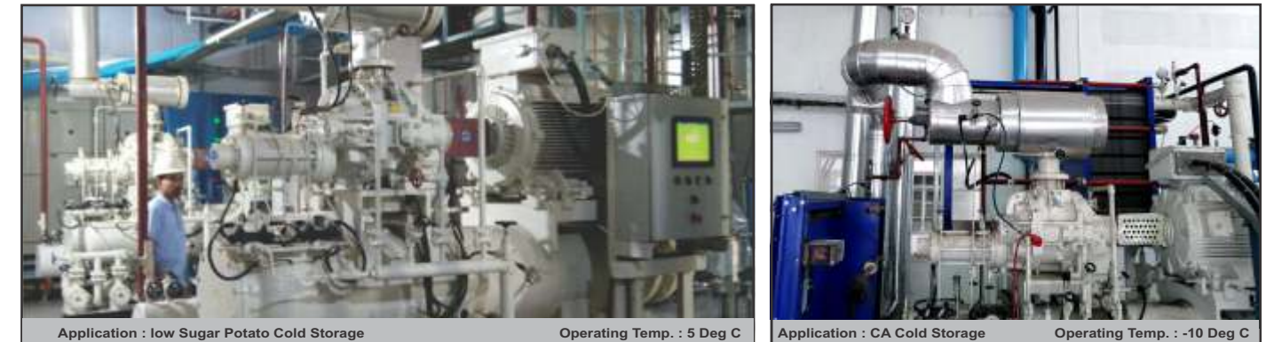
Application : low Sugar Potato Cold Storage Operating Temp. : 5 Deg C
